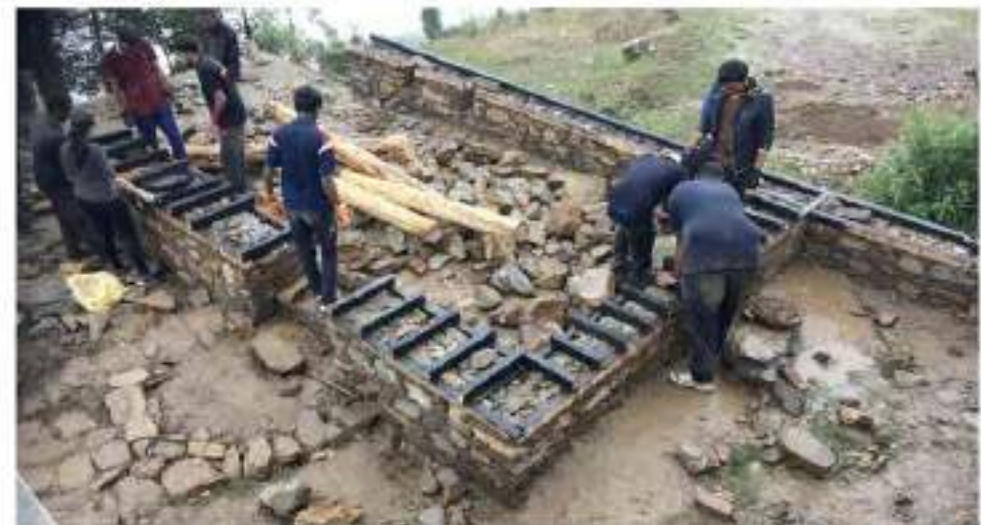
wooden bands for earthquake resistance
